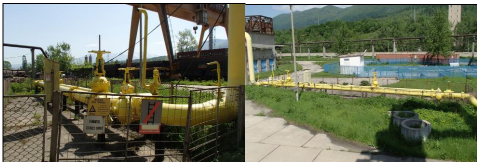
Fig.3. The measurement regulation station
